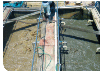
Operation in a aeration tank running condition
