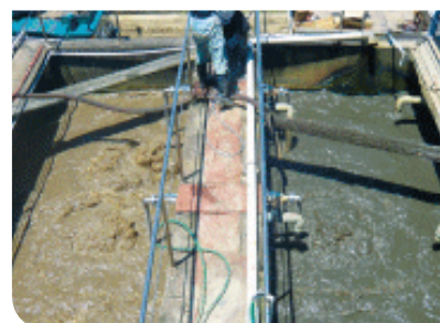
Operation in aeration tank running condition
